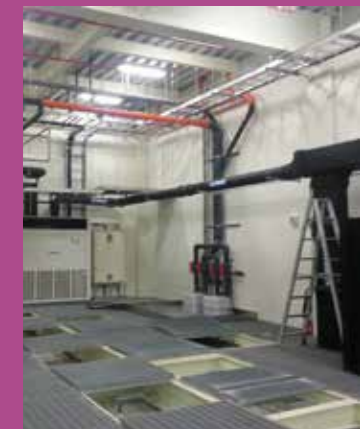
Two SANICUBIC® 2 Pro Installed in the basement to remove waste water
