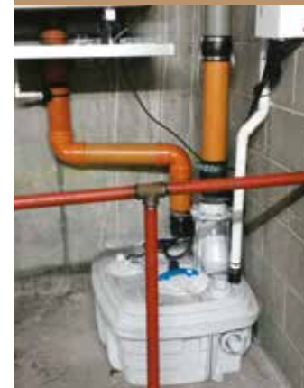
SANICUBIC® 2 XL Installed in the technical room
