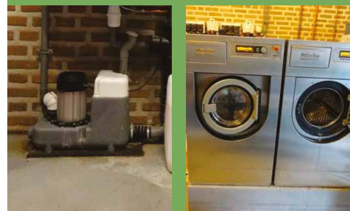
SANICOM® 1 lifting pump installed in the basement
