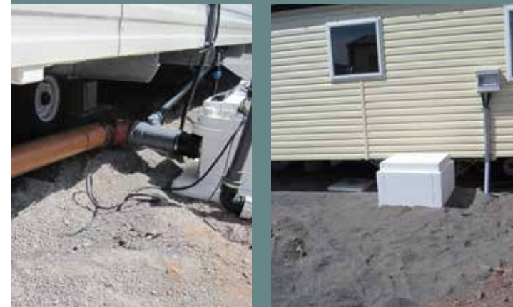
SANICUBIC® 2 Pro lifting station installed
